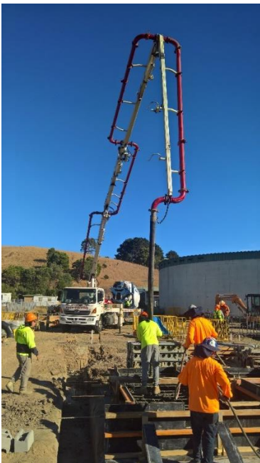
Pump station and dosing facility construction at the Lance Creek Water Treatment Plant
