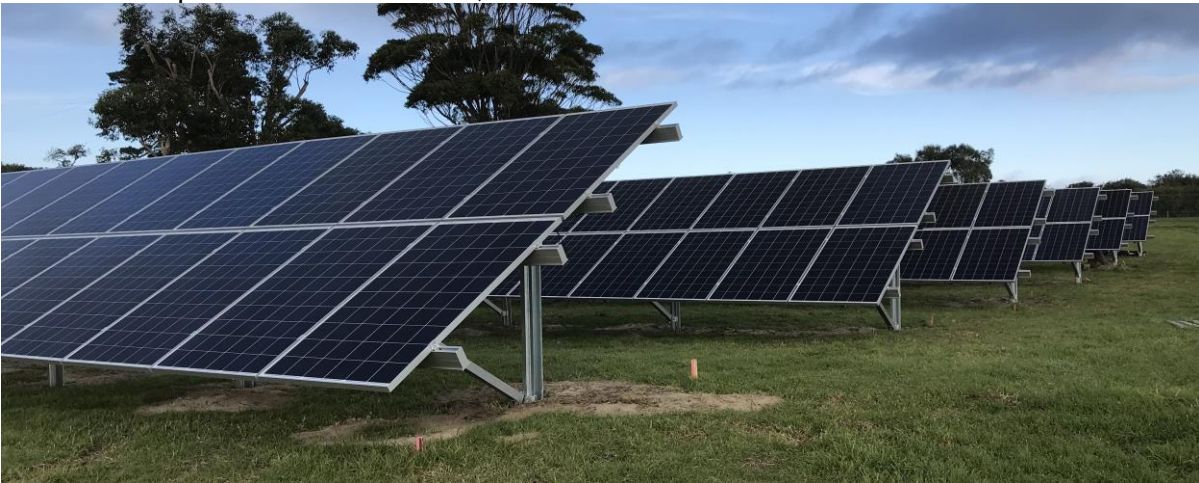
6 banks of panels make up the 75.6 kW system
