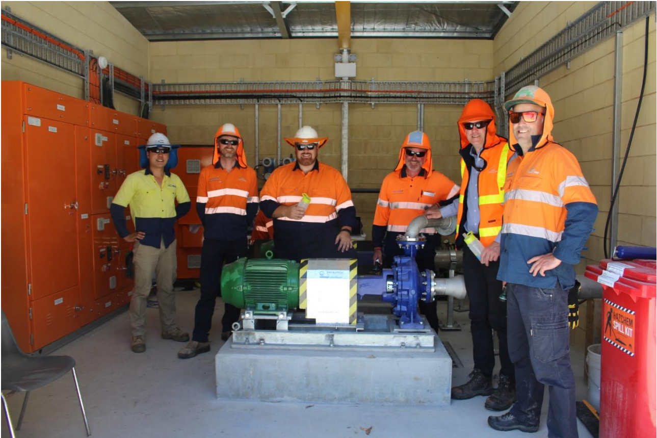
Members of the Lance Creek Water Connection project team with the newly commissioned pumps that will transfer an average of 800 KL water per day from Korumburra to Poowong. L:R Simon Chen Simpson Construction Company . Chris Hindle, Nathan Lucas, Glen Baldwin, Mark Lynch and Dean De Menech of South Gippsland Water
