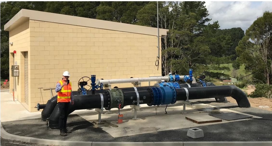
Mark Lynch, General Manager Infrastructure & Planning, South Gippsland Water, Standing in front of the pipeline and pump station at Korumburra
