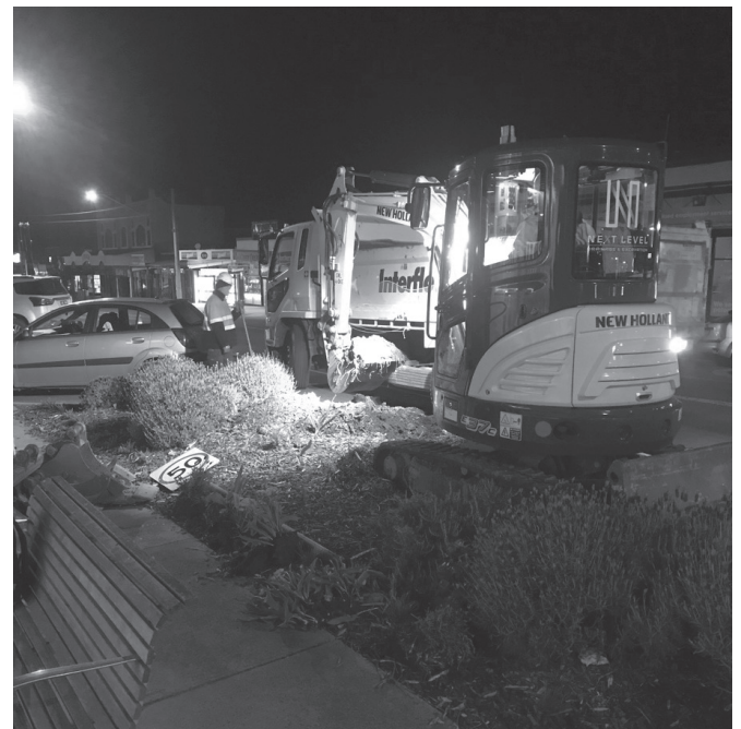
Night works to upgrade 100 year old water main. Sep 2019 - Graham St, Wonthaggi
