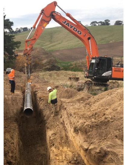
Milestone - final section of steel pipe in the Lance Creek to Korumburra portion of the pipeline was installed 24/04/2018
