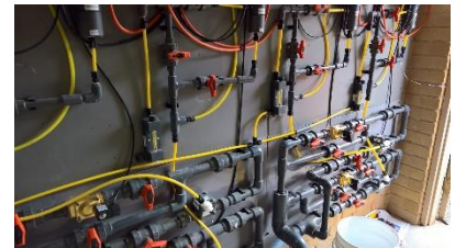
New chemical dosing infrastructure.
