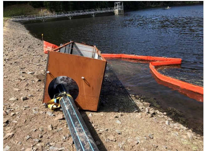
Water being released into Little Bess Reservoir as pipeline and pumps are tested this week.
