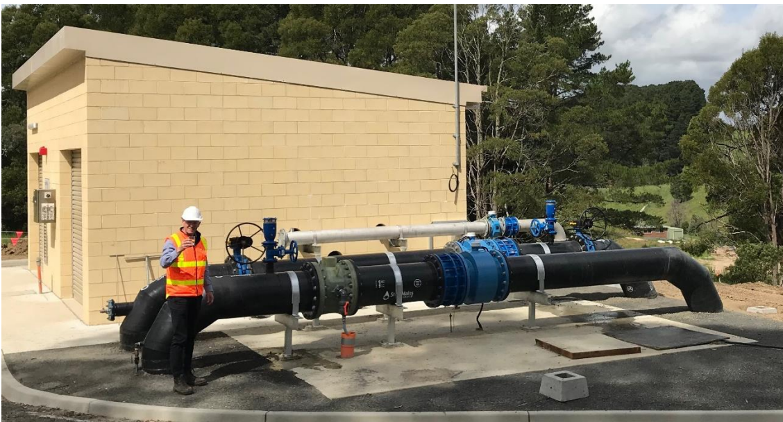
Mark Lynch, General Manager Infrastructure & Planning, South Gippsland Water, Standing in front the pump station at Korumburra – these pumps will transfer an average of 800KL water per day to Poowong.
