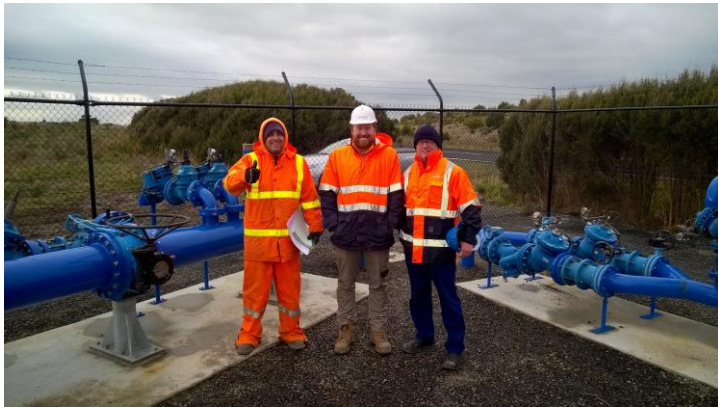
Commissioning of DP5 valve which connects Lance Creek Reservoir to the Desalination Plant and Melbourne Water Supply System.
